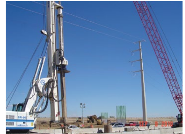
Daily activity looking east from the west end of the jobsite at Academy Blvd. and Drennan Rd.
